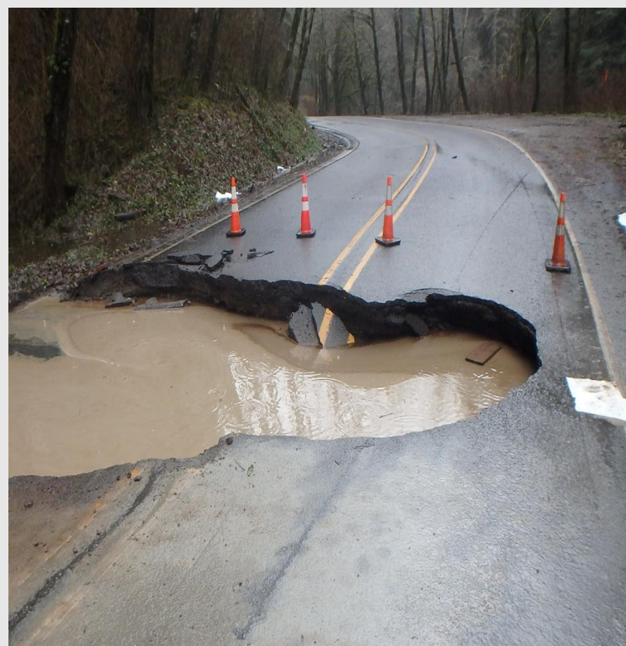
Extreme Rain, Snow and Flooding
