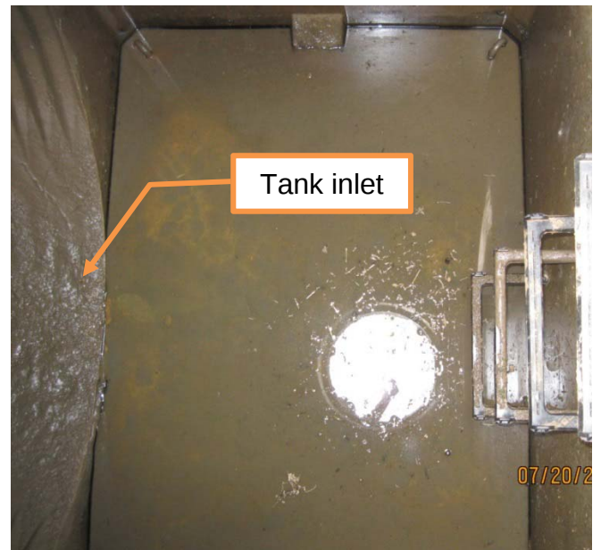
Figure 10: Interior view of access vault
