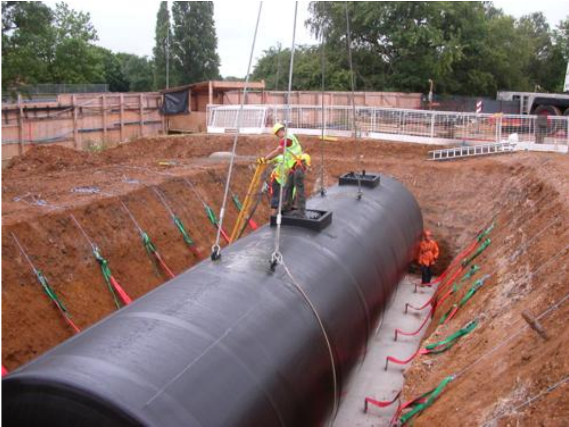
Figure B-12: Main tank (T8)
