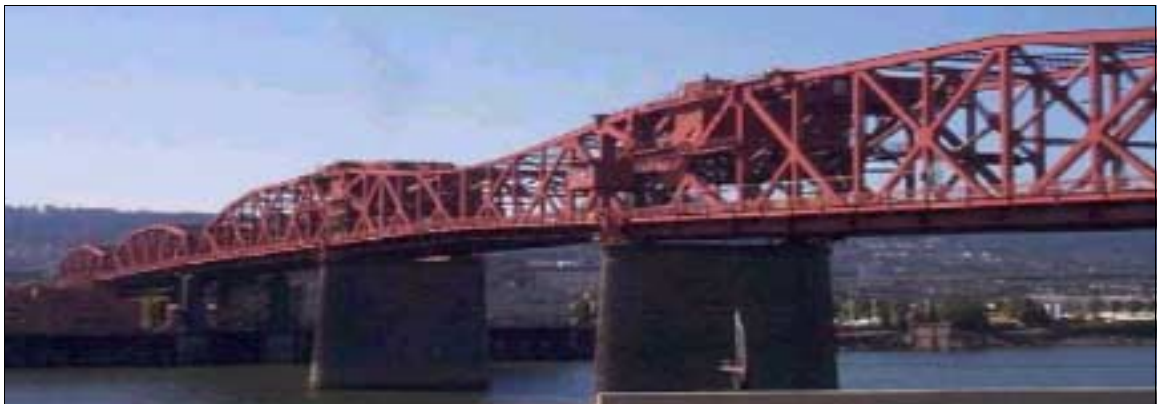
Broadway Bridge spans the Willamette River in Portland. Bridges are critical lifelines. (photo courtesy of Multnomah County)
