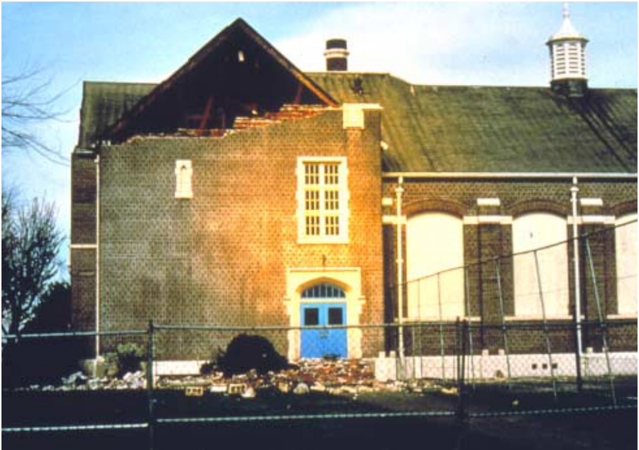
Molalla High School was condemned after the 1993 Scotts Mills earthquake (M5.6). A new high school was built on another site. (photo courtesy Oregon Department of Geology and Mineral Industries)
