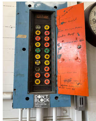
End of life fuse box
