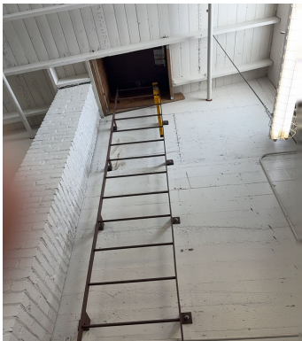
Unsafe roof access
