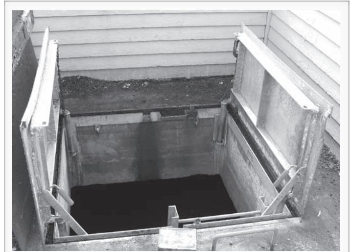
Gutter hatch = example of hatch no longer accepted
