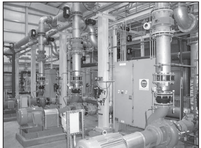
Finished water pumps and plant piping. Membranes located in basin in background.
