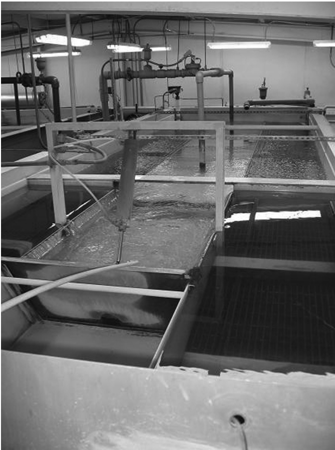
Creswell's old clarifier and filters.
