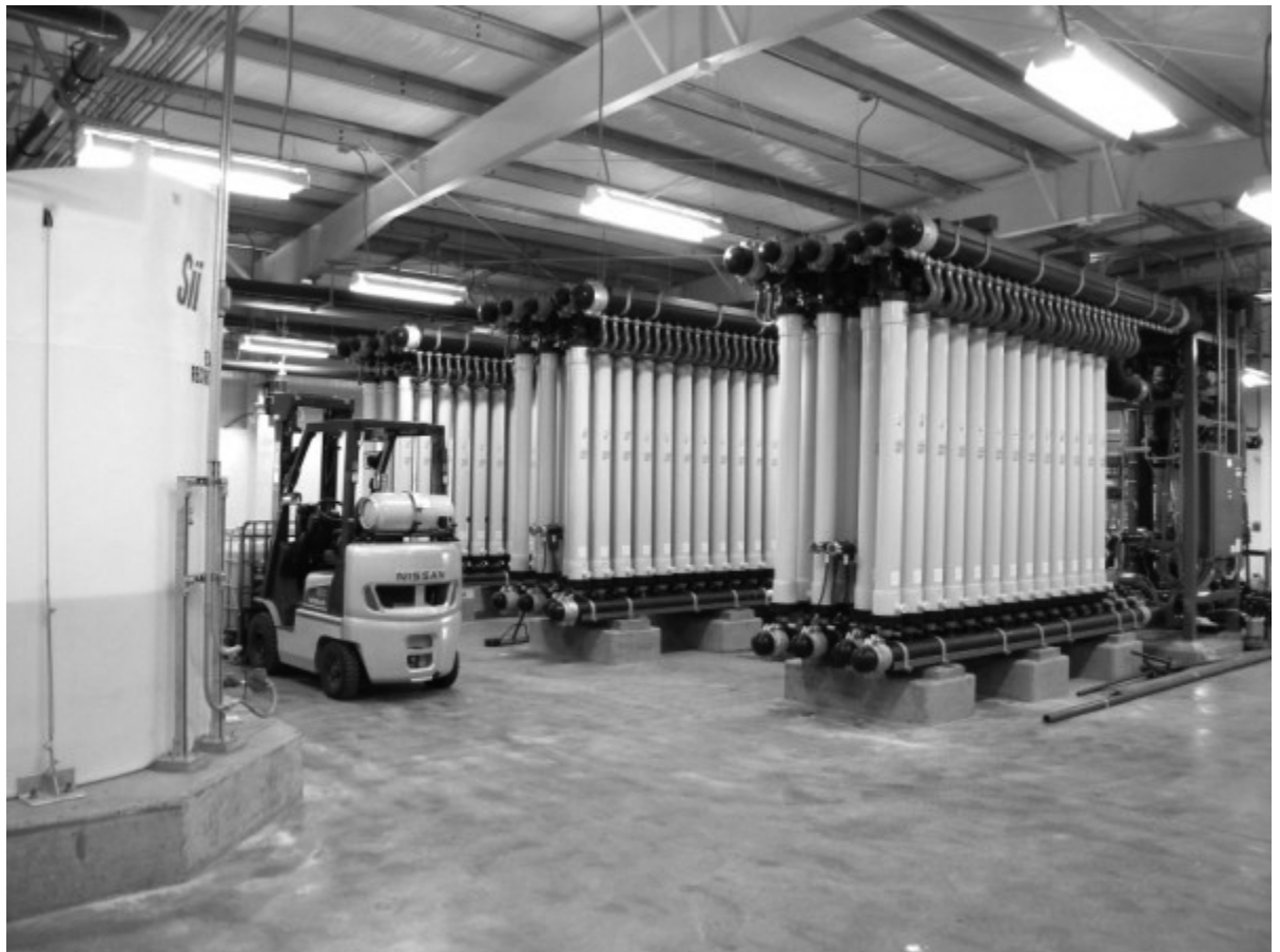
Creswell's new membrane filtration plant.
