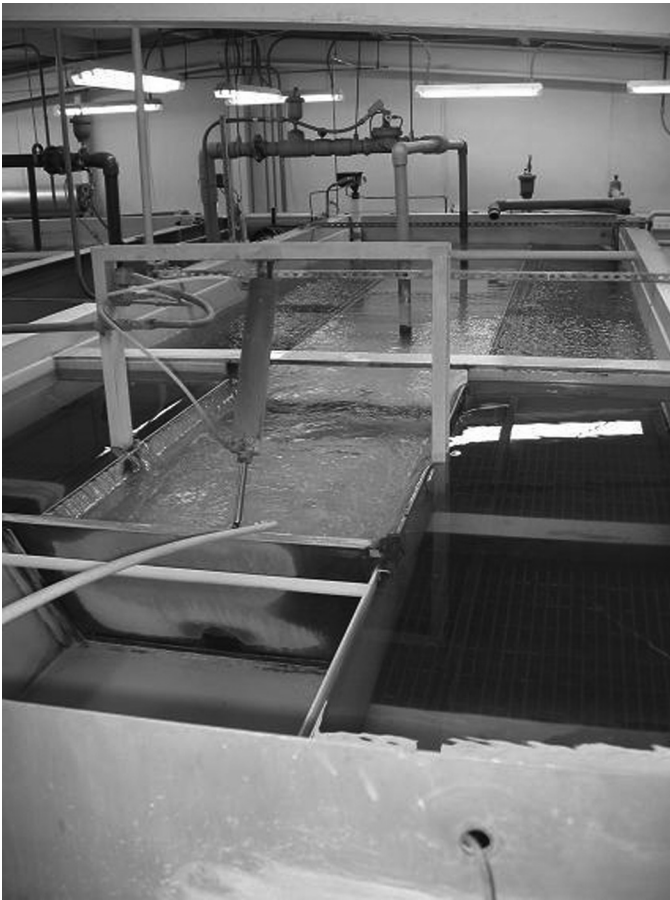
Creswell's old clarifier and filters.
