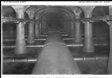
J. MAIN COLLECTOR AND LATERALS BEFORE SAND AND GRAVEL WERE PUT IN.
