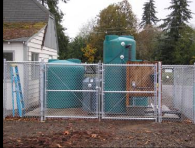
2009. Jewell School District #8, OR. "Blue Future" covered filter (left) and raw water control tank (right)
