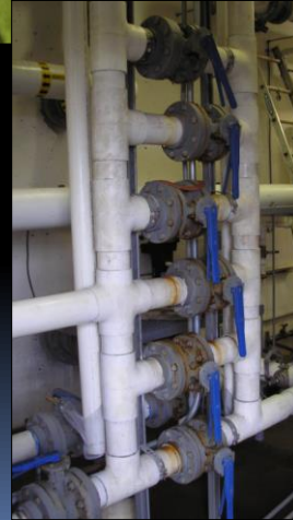
Butterfly valves. City of Banks in Washington Co. Oregon. 2011.
