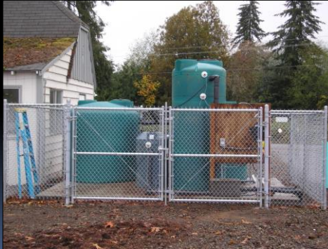
2009, Jewell School District #8, OR. "Blue Future" covered filter (left) and raw water control tank (right)
