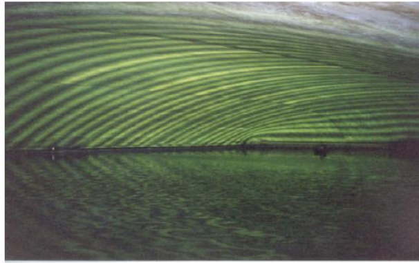
Plate 2.2 - Internal view of a slow sand filter covered by plastic film supported by positive air-pressure at Walton, Thames Water
