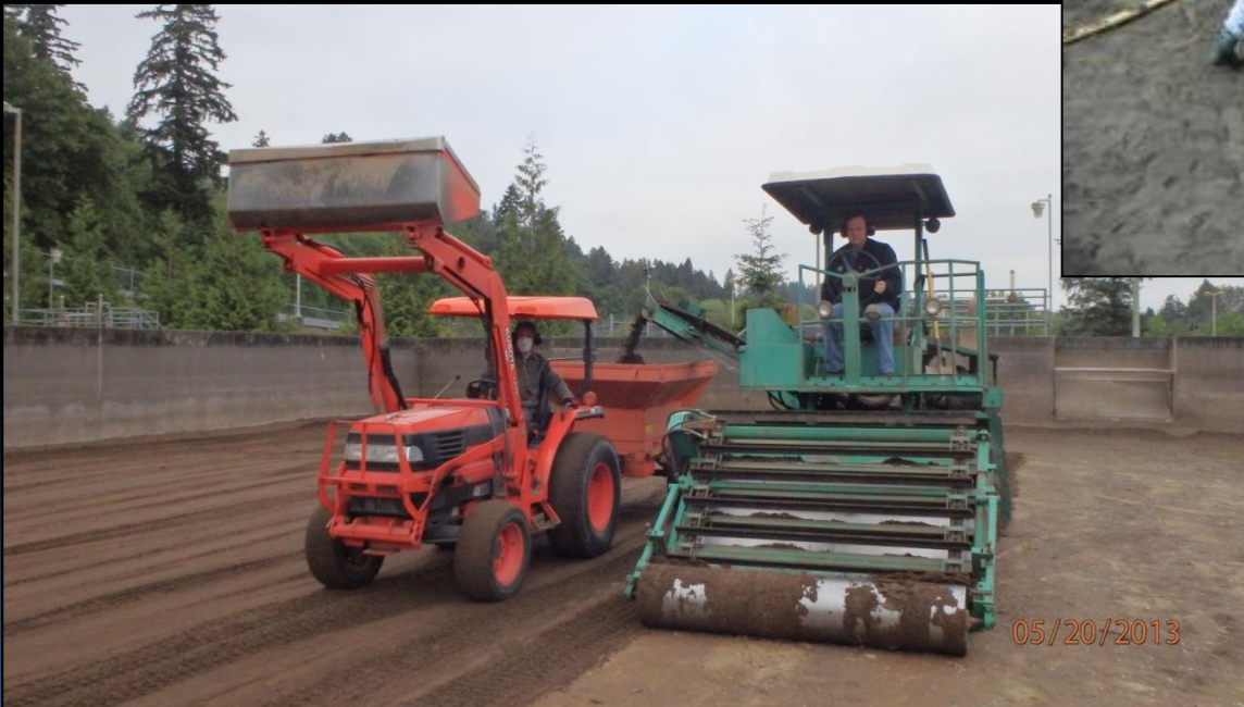
2013. North Clackamas County Water Commission, OR. SSF Cleaning (photo taken by Chris Johnsen, NCCWC)
