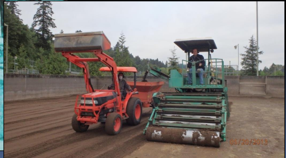
2013. North Clackamas County Water Commission, OR. SSF Cleaning (photo taken by Chris Johnsen, NCCWC)
