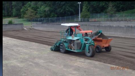
2023, North Clackamas County Water Commission, OR. SSF Cleaning (photo taken by Chris Johnson, NCCWQ)
