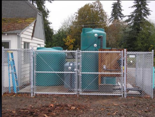
2009. Jewell School District #8, OR. "Blue Future" covered filter (left) and raw water control tank (right)
