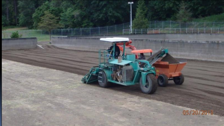
2013. North Clackamas County Water Commission, OR. SSF Cleaning (photo taken by Chris Johnsen, NCCWC)
