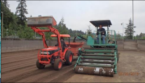
2013, North Clackamas County Water Commission, OR. SSF Cleaning (photo taken by Chris Johnsen, NCCWC)
