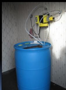
Diaphragm pump with chlorine solution tank
