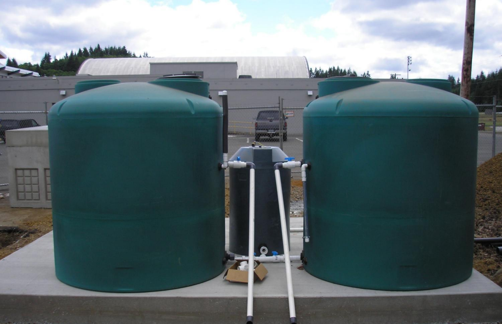
Self-contained slow sand filters at a school designed for wet harrowing.
