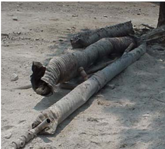
Figure 9: Asbestos-Containing Steam Pipe
