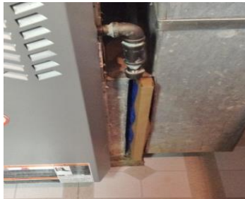
Open filter slots must have new covers installed
