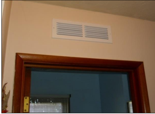
Through the wall bypass grille
