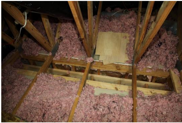
Seal top of soffit: Before- Wall cavities are open to the attic allowing for air leakage into the attic.
