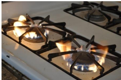
Uneven luminous flames are a sign that the burners require servicing.
