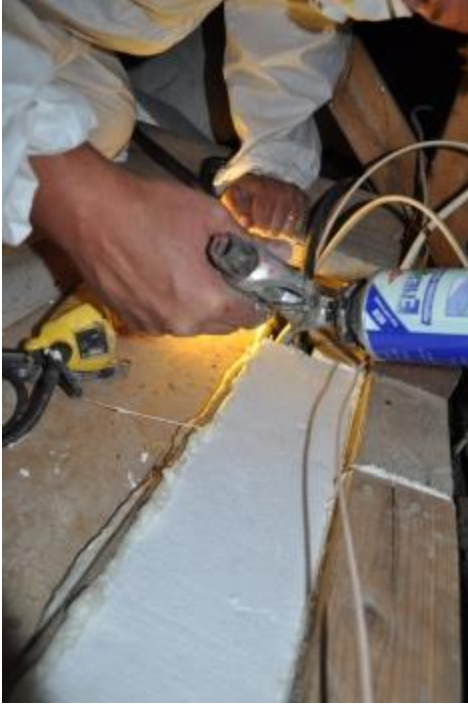
Sealant must be used to fill in all cracks and gaps along the edges of the chase cap
