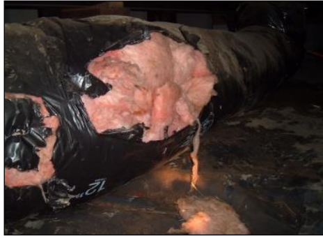
Damaged Flex Duct
