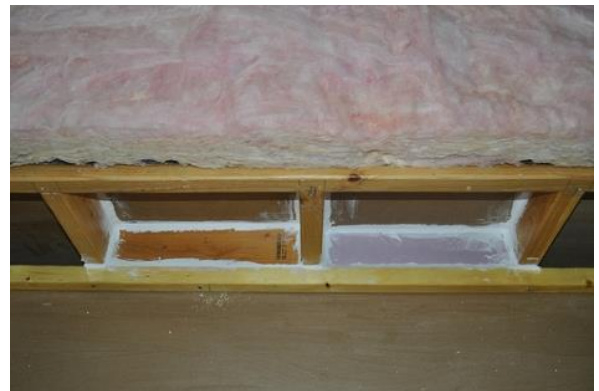
Option 1: Span each stud bay with rigid material at the level of the stud bay, seal thoroughly.
