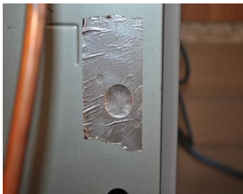
Foil tape should be used to seal all holes in air handler cabinets
