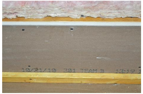
Option 3: Stud bay will be covered with rigid material, fastened and sealed.
