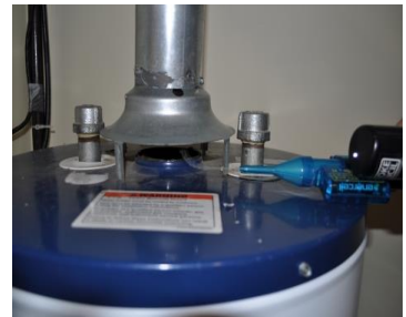
Test for spillage using chemical smoke or a mirror.
