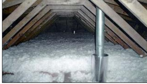
Shielded B Vent in Attic
