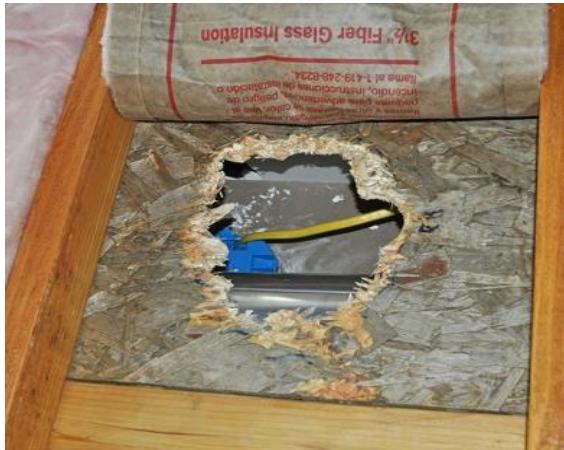
Prepare work area by removing existing insulation and debris from top ceiling
