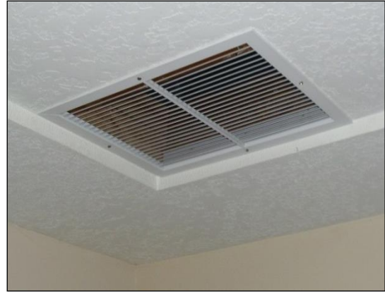
Ceiling jump-over duct grille
