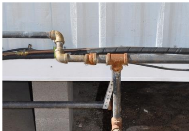
Inspect exterior fuel lines for leaks or damage.
