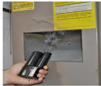
On natural draft furnaces, test for spillage on all sides of the draft
