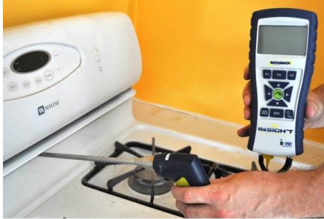
Test for CO in the oven exhaust port
