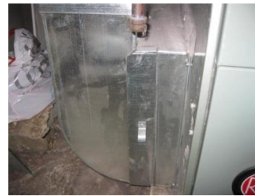
A properly fitting filter slot cover prevents garage pollutants from entering the conditioned space
