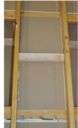
Once the chase is capped, the joint along the framed must be sealed
