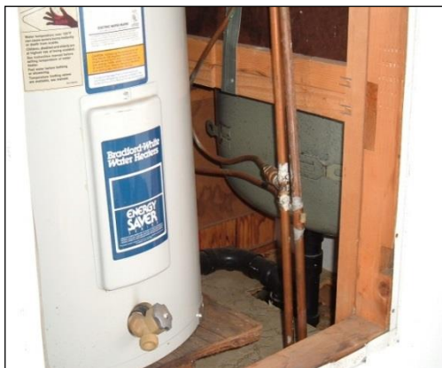
Water heater/bathtub penetration
