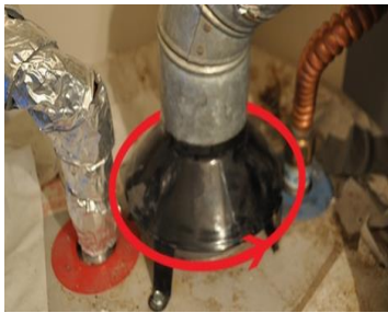
On water heaters, test for spillage on all sides of the draft diverter
