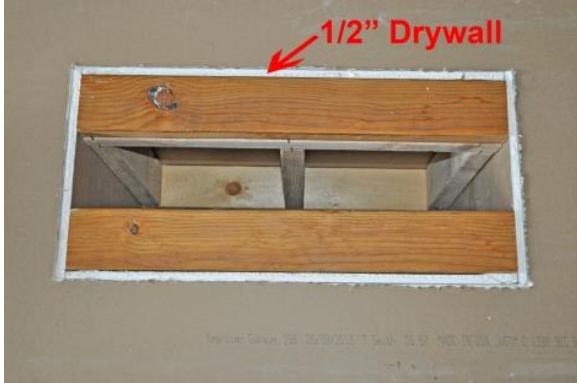
Clear area of insulation and debris
