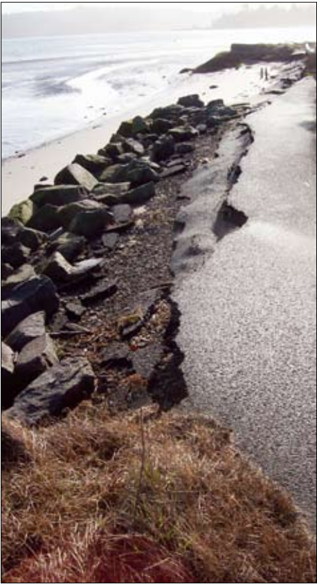
Above: A view of some of the erosion and damage to the Hatfield Marine Science Center’s coastal estuary trail in Yaquina Bay in Newport, Ore. Oregon Soldiers worked on a project to mitigate some of the beach erosion and restore sections of the trail in March, 2007.
