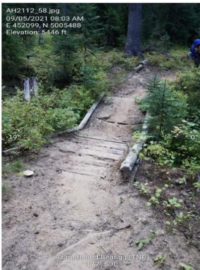
Figure 9, Bridge on ~7060 North Fork Catherine Creek with 8 failed log stringers
