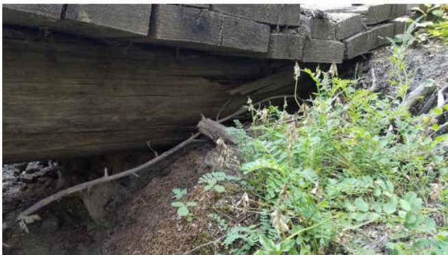
Figure 8, Detail of bridge on ~7066 West Fork Wallowa showing rotten-broken stringer log.
