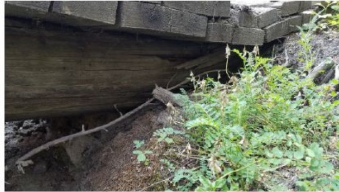
Figure 8, Detail of bridge on ~7066 West Fork Willows showing rotten-broken stringer log.
