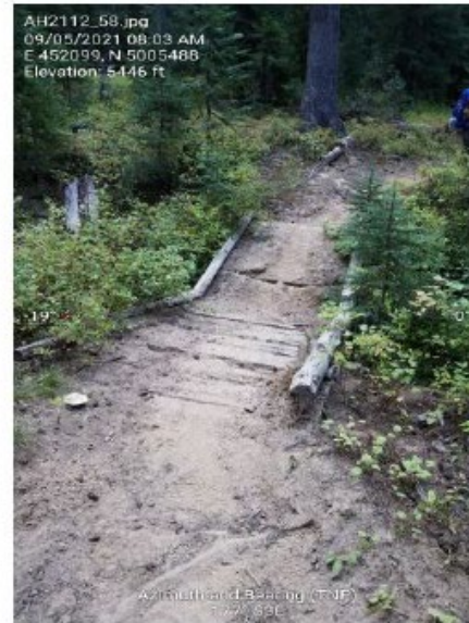
Figure 9, Bridge on ~7060 North Fork Catherine Creek with failed log stringers
