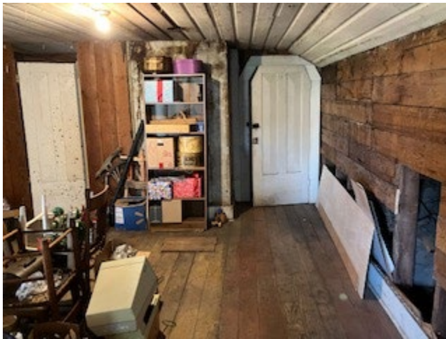
Unique doors will be preserved, Floor wall markings are evident in this room.
