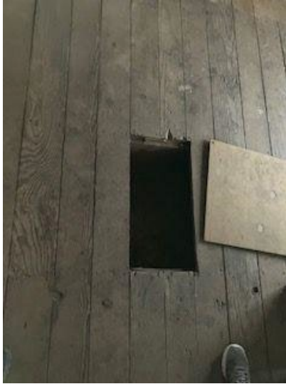
One of holes in the floor that will be fixed.
