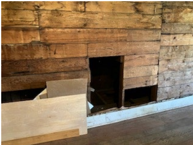
An appropriate entrance to the attic space will be created and covered for safety. This shows the access point to one of the future HVAC units.
