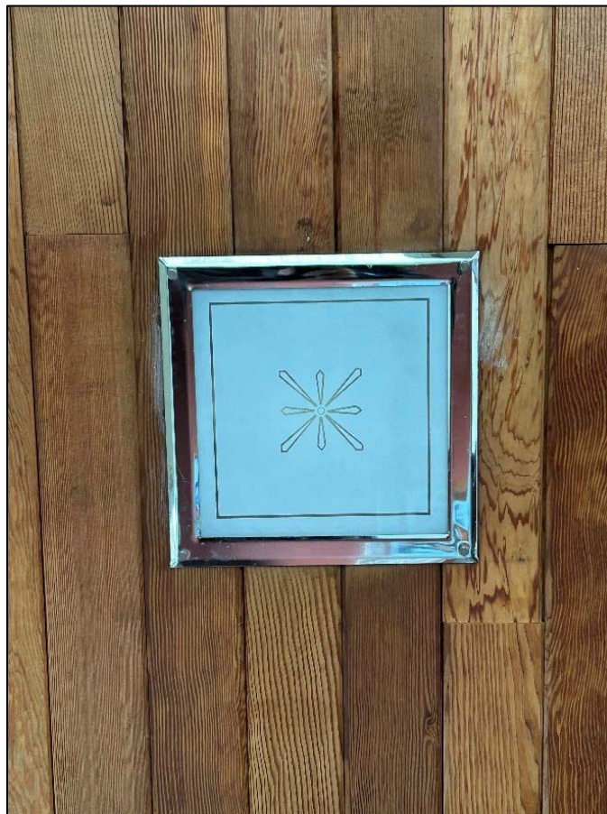
Photograph 4 of 16: OR_BentonCounty_YangEdithHouse_0004 An original recessed ceiling light, found throughout the Edith Yang House, including in the entry courtyard.
