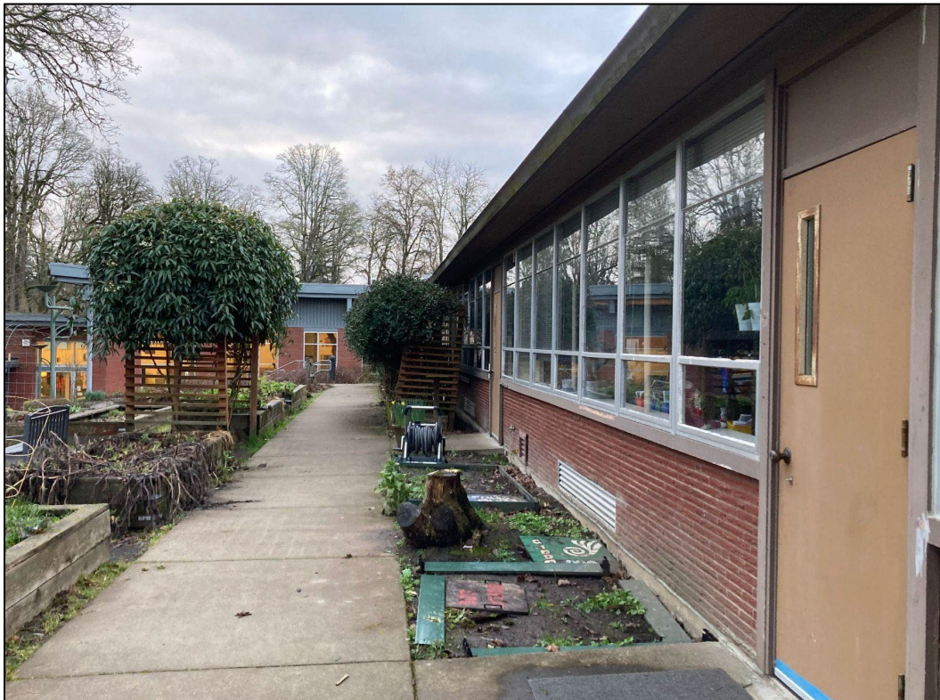
Photograph 8 of 15: OR_ClackamasCounty_BoltonSchool_0008 Looking northeast along rear (northwest) elevation, classroom wing with ribbon windows and teaching garden. Library addition at left.
