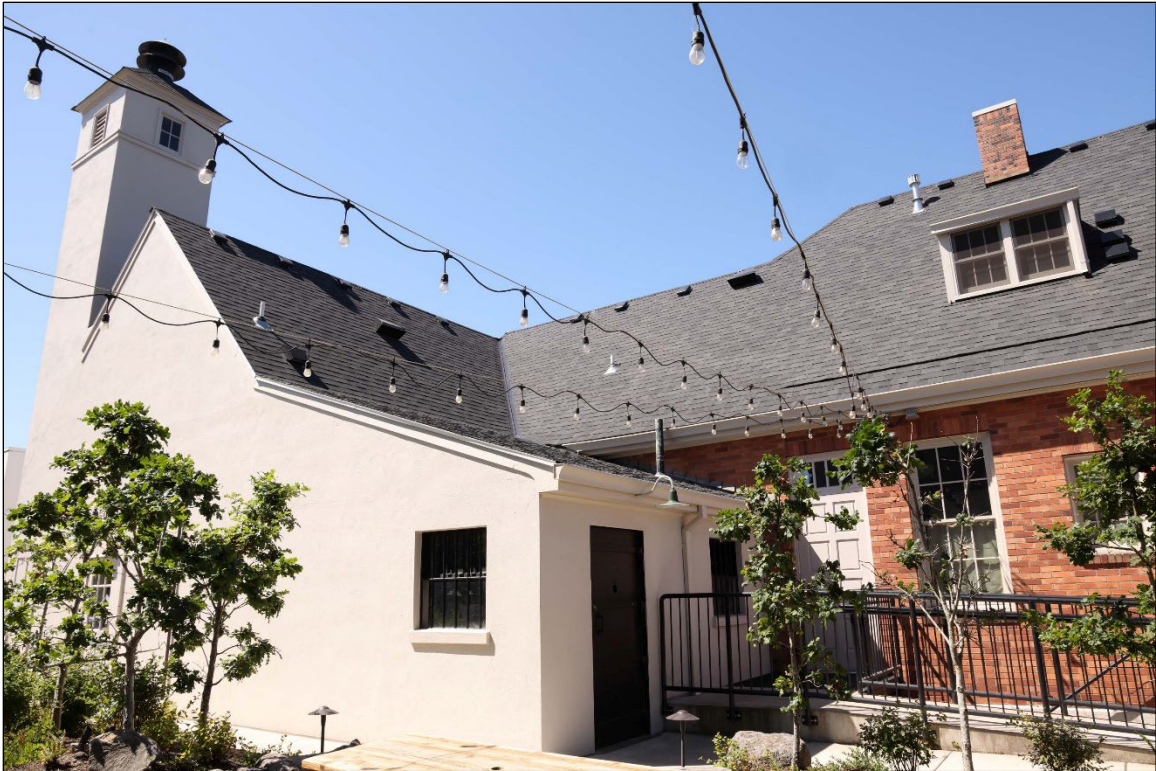
Photograph 7 of 14: OR_ClackamasCounty_CanbyCityHall_0007 Oblique view of east façade centered on the jail, camera facing south-southwest.
