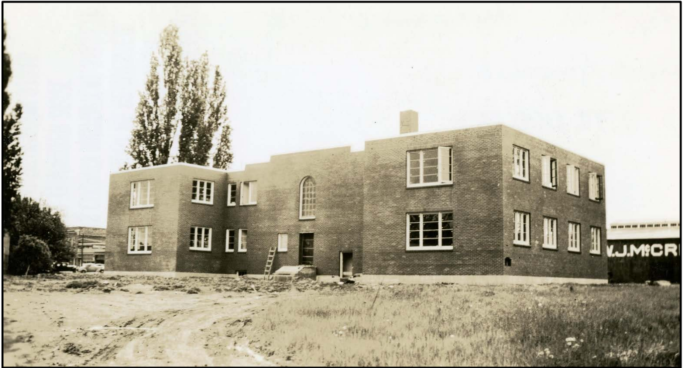
Figure 12. Rear (east) side of the new Milwaukie City Hall during construction in 1938. Source: Clackamas County Historical Society, P-320.
