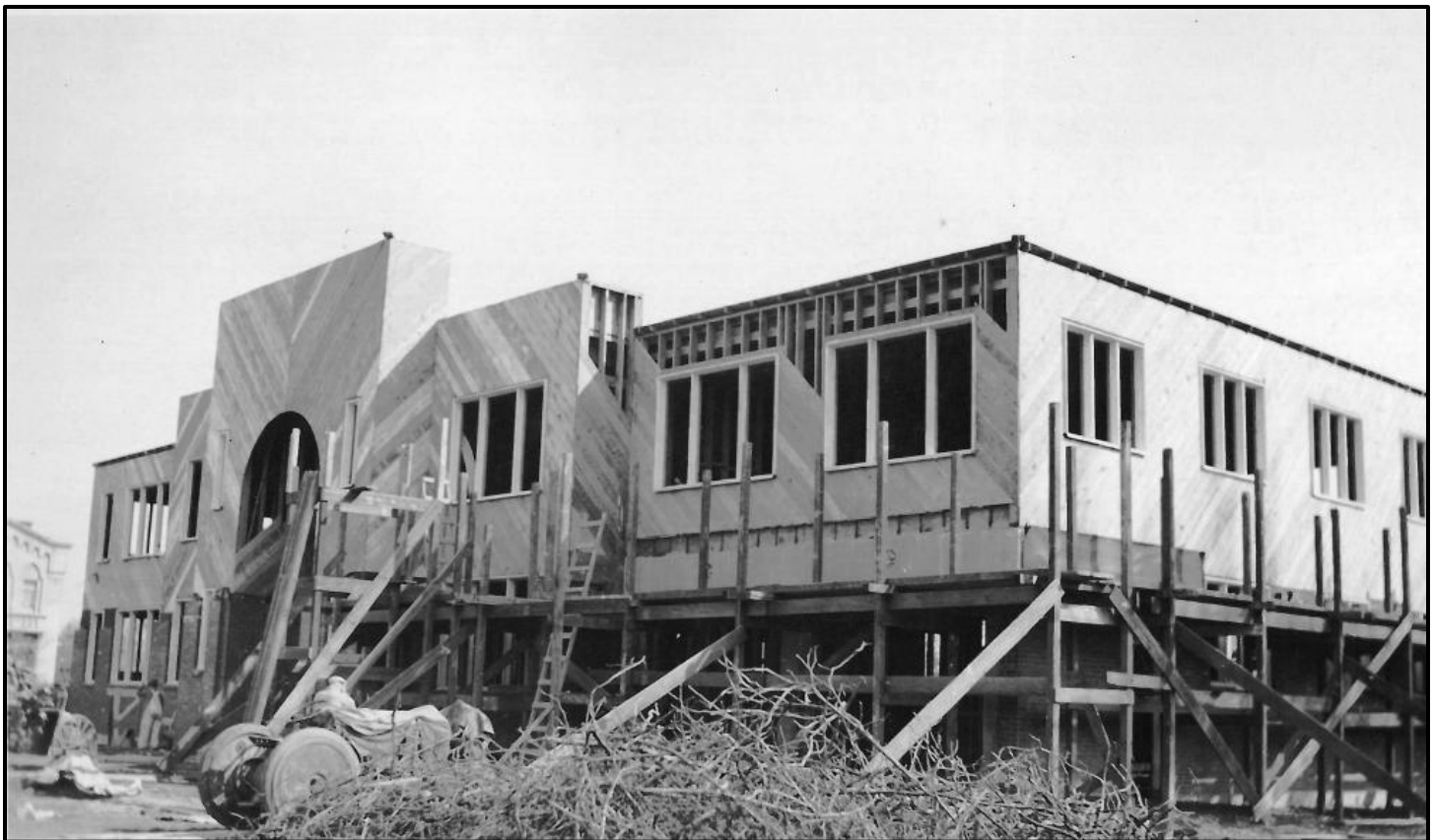
Figure 11. Front (west) side of the new Milwaukie City Hall during construction (1938). Source: City of Milwaukie.
