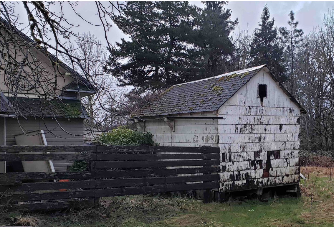
Photo 24. Francis and Helen Nordstrom fruit cellar, north side and west (rear) elevations, looking southeast.
