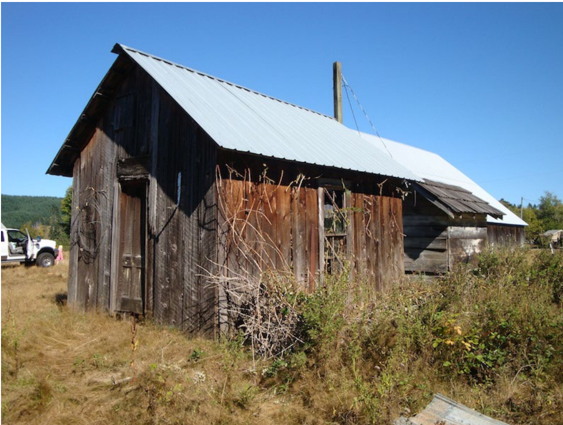
Photo 16. Shop, west and south elevations, view looking northeast with pump house behind.
