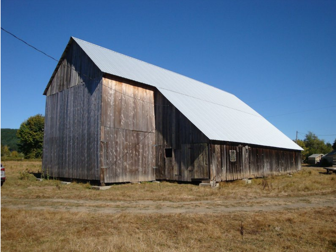
Photo 9. Cahill-Nordstrom barn, west and south sides looking northeast, with drive-through hay shed at left.
