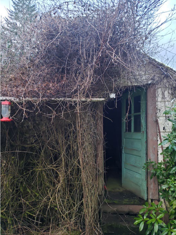
Photo 23. Francis and Helen Nordstrom fruit cellar, front wall and entrance (east end), looking west.
