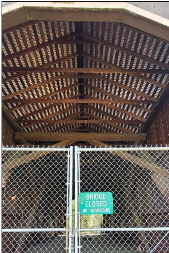
Photograph 8 of 9: OR_DouglasCounty_PassCreekCoveredBridge_0008 Top of wood Howe truss and roof framing inside Pass Creek Covered Bridge, camera facing south.
