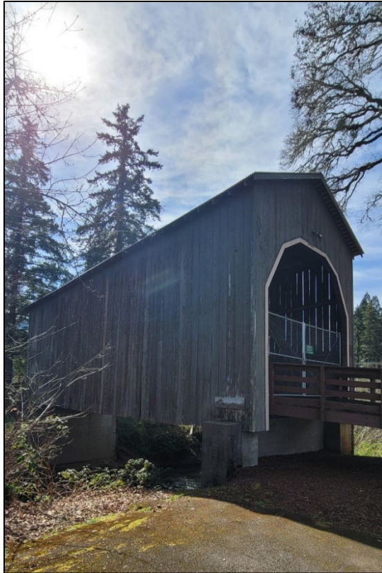
Photograph 5 of 9: OR_DouglasCounty_PassCreekCoveredBridge_0005 East wall and north portal of Pass Creek Covered Bridge, camera facing southwest.
