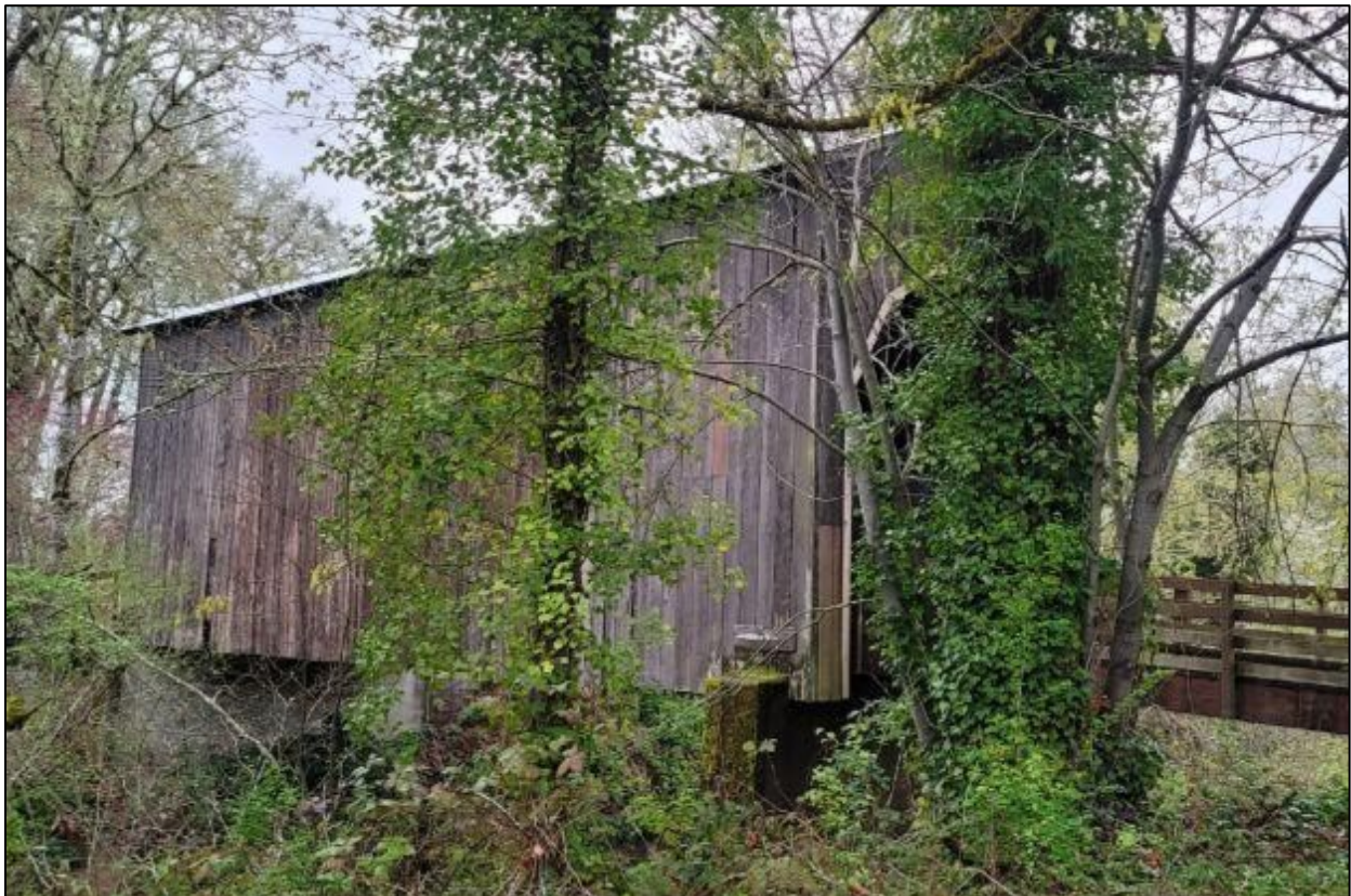
Photograph 2 of 9: OR_DouglasCounty_PassCreekCoveredBridge_0002 West wall and south portal of Pass Creek Covered Bridge, camera facing northeast.
