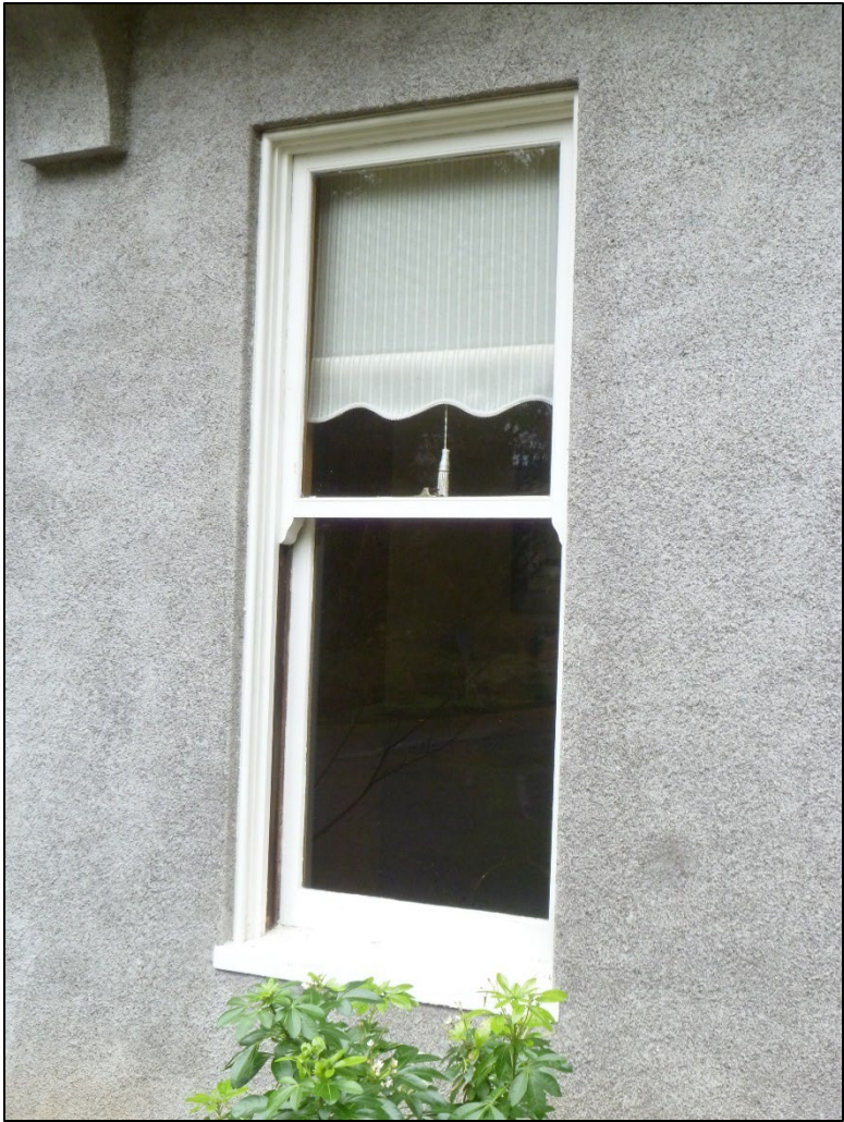
Figure 23: Recessed window on Kerr house, built 1917. Photo taken February 2026, Eileen G. Fitzsimons.
