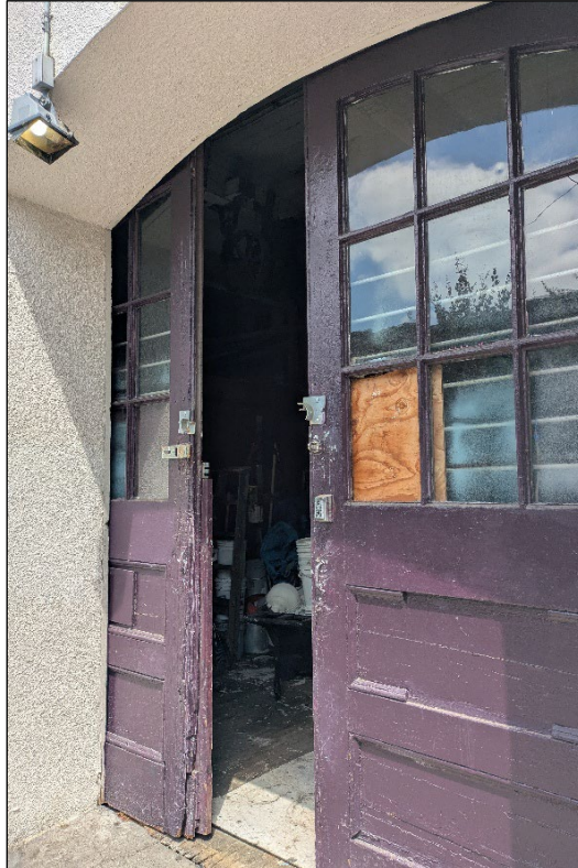
Photograph 6 of 15: OR_MultnomahCounty_OregonCasketCompanyBuilding_0006 The original double loading door on the south elevation; camera facing northwest.
