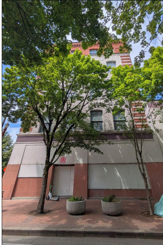
Photograph 2 of 15: OR_MultnomahCounty_OregonCasketCompanyBuilding_0002 East elevation with door and windows from the 1954 renovation boarded up since 2020; camera facing west.
