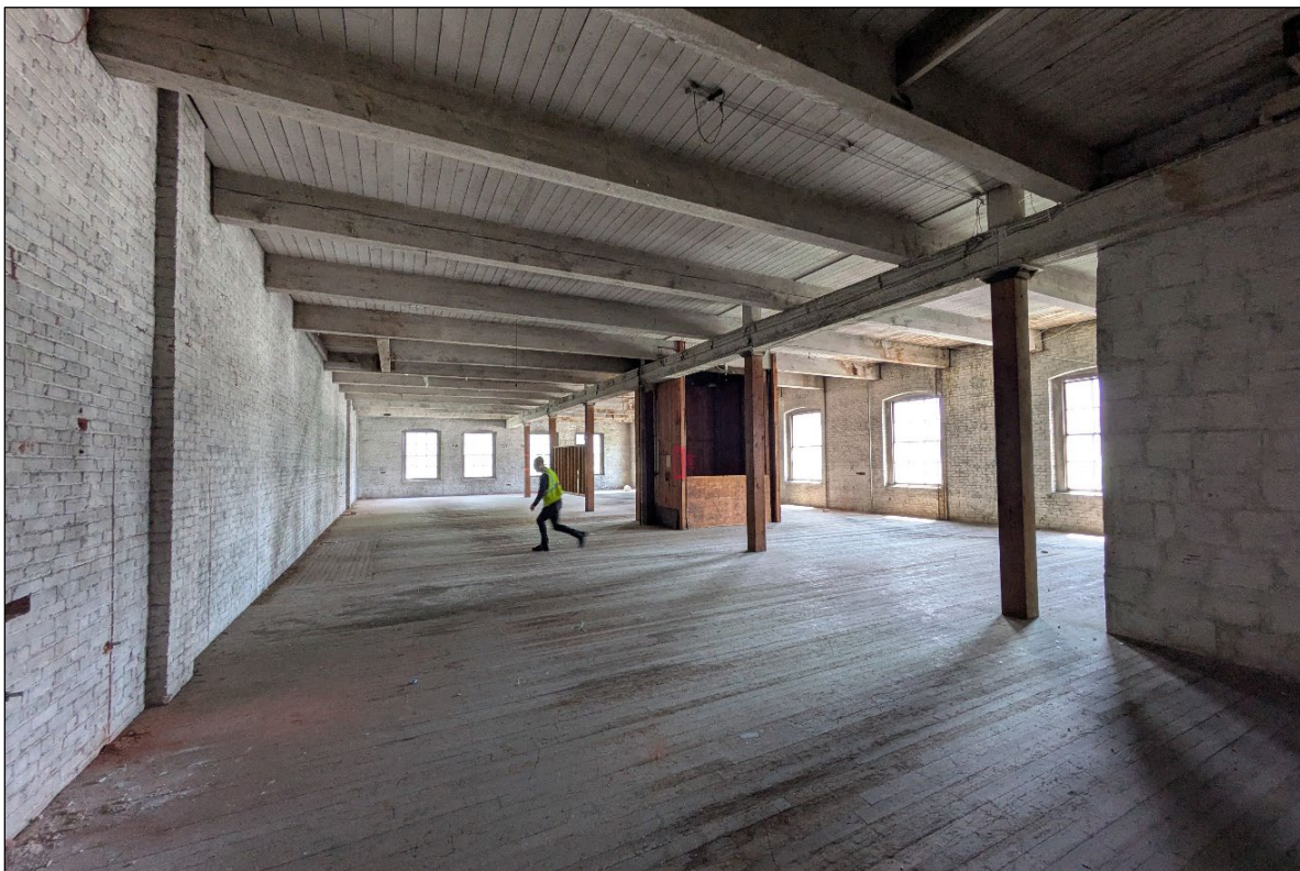
Photograph 12 of 15: OR_MultnomahCounty_OregonCasketCompanyBuilding_0012 Third floor showing elevator at middle and staircase enclosure at right; camera facing southeast. Ghost marks on the left wall and framing modifications at the ceiling indicated the location of an older staircase.
