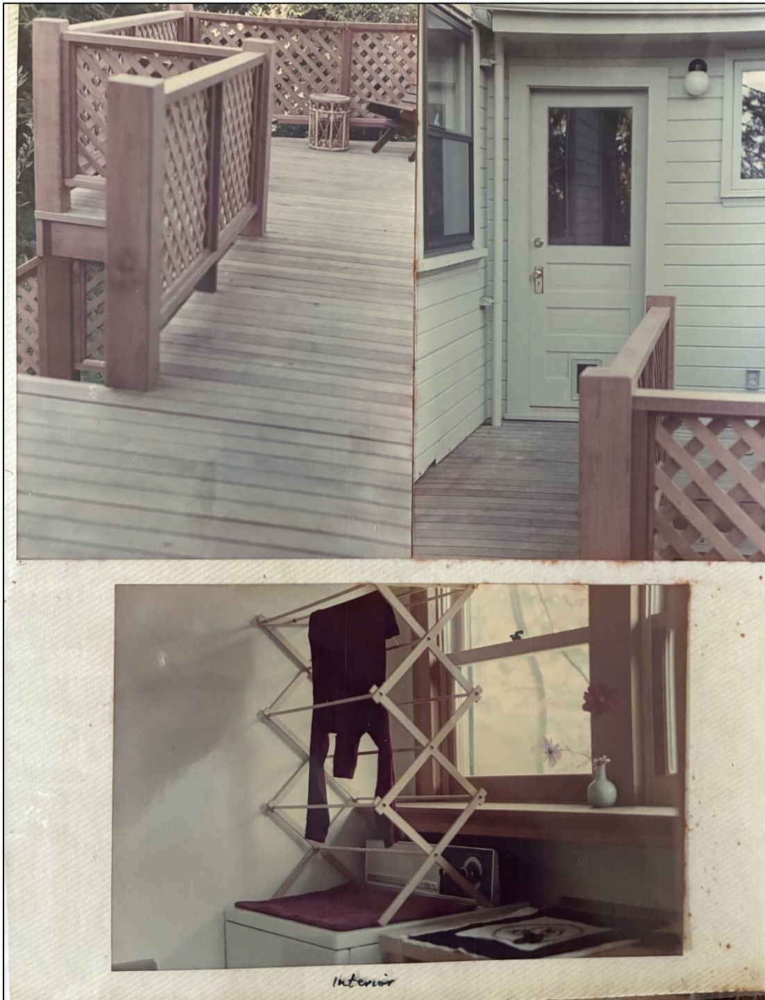
Figure 14: Construction photos showing 1984 deck and Laundry Room Addition at the west side of the house. Source: Le Guin Family Collection.
