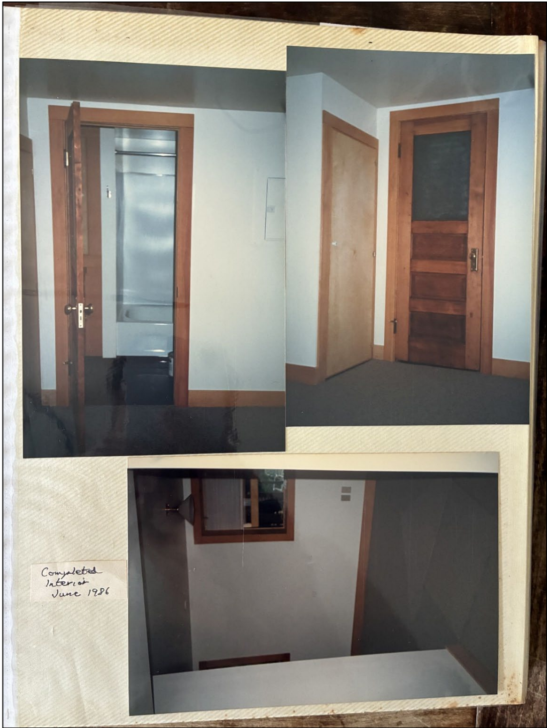
Figure 20: Basement apartment unit construction photos, 1986. View looking northeast at west elevation. Source: Le Guin Family Collection.
