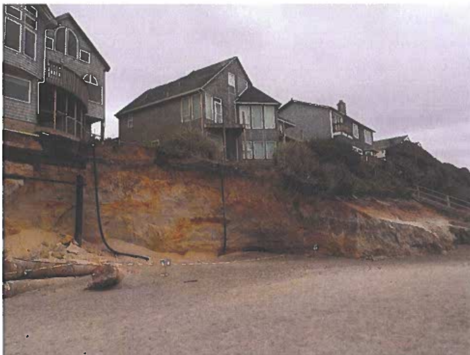
Photo 3 – Southeasterly view of the bluff slope fronting Tax Lot 14900. The recent severe erosion undercut the more resistant gray sandy silt and rapidly eroded the underlying weakly cemented sand. Photograph taken August 17, 2021.
