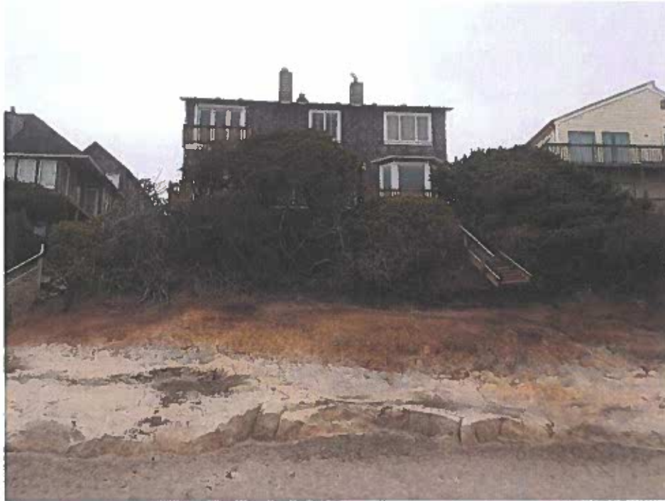
Photo 1 – Easterly view of the bluff slope fronting Tax Lot 14800. Note the wooden access stairs are hanging above the slope and the erosion scarp at the toe of the slope. Photograph taken August 17, 2021.
