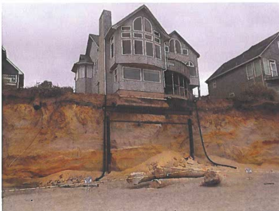
Photo 4 – Easterly view of Tax Lot 15000. The recent severe erosion undermined the house foundation, and new pile supporting the foundation were installed to prevent damage or collapse of the house. Photograph taken August 17, 2021.
