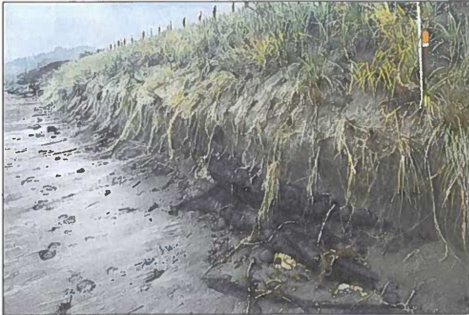
Photo 6: Site conditions at 3188 Pacific Avenue on November 21, 2024, showing the eroded planting media, damaged soil burritos, and oversteepened (~0.5H:1V) eroding bluff slope shortly after reconstruction in summer 2024.
