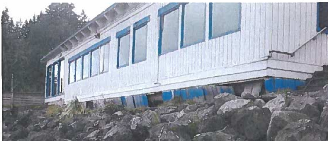
Figure 4. Damage by overtopping waves reaching a building (Discovery Bay, 2025)
