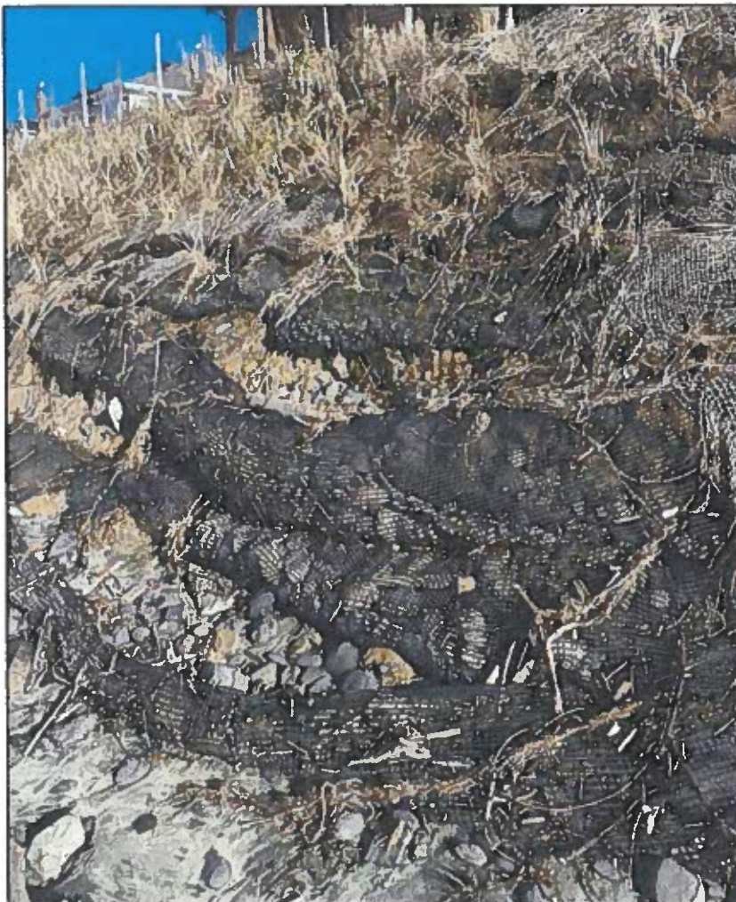
Photo 5: Site conditions at 3188 Pacific Avenue on September 8, 2022 showing the damaged vegetated soil burritos that required reconstruction.
