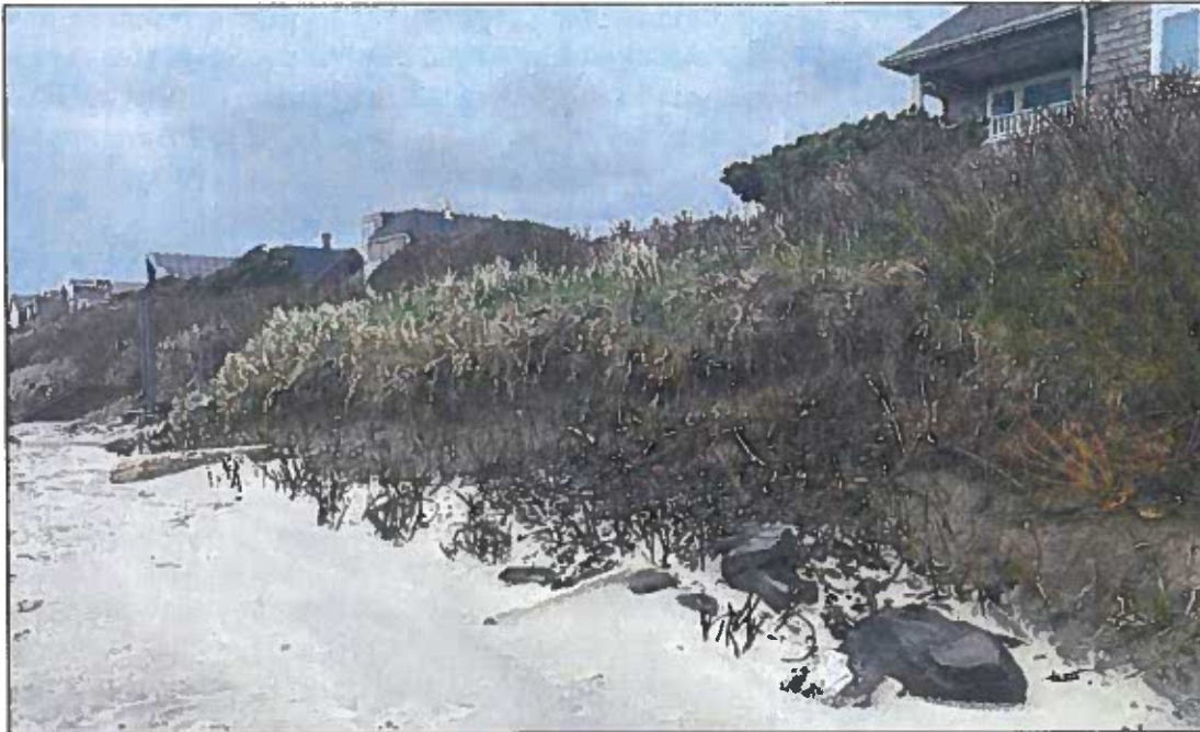
Photo 3: Site conditions observed during our initial visit on April 20, 2023, showing active erosion along the approximately 4- to 7-foot-tall bluff. Trace amounts of cobbles and angular rock placed at the toe of the bluff are also visible.
