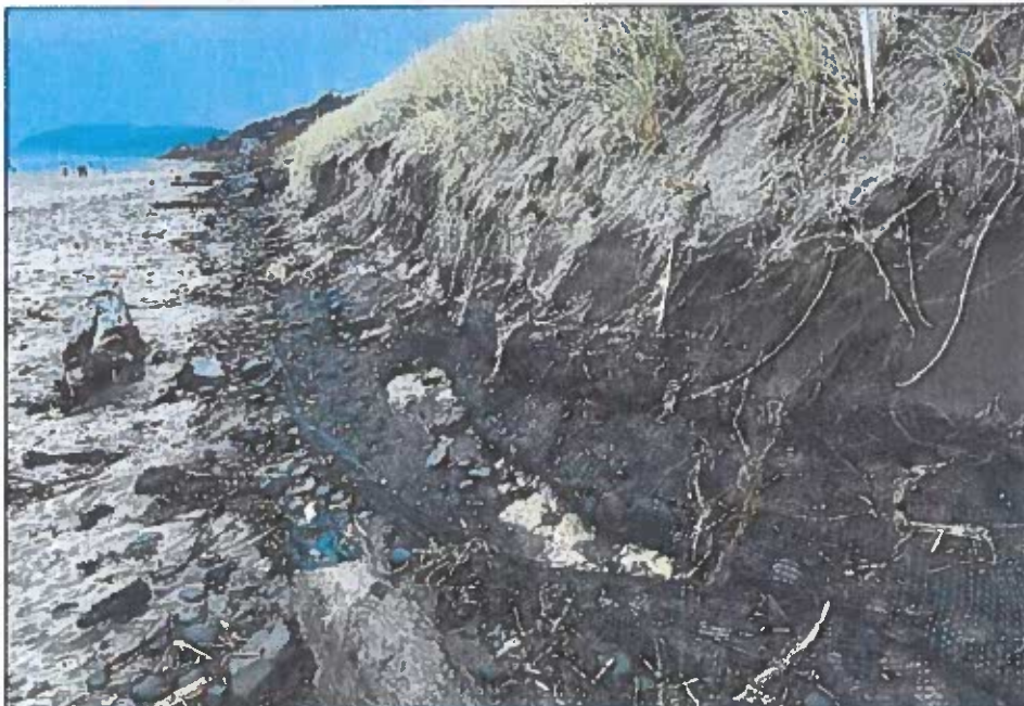
Photo 7: Site conditions at 3188 Pacific Avenue on December 16, 2024, showing the rapid erosion occurring at the base of the bluff slope less than one month after Photo 6 was taken.
