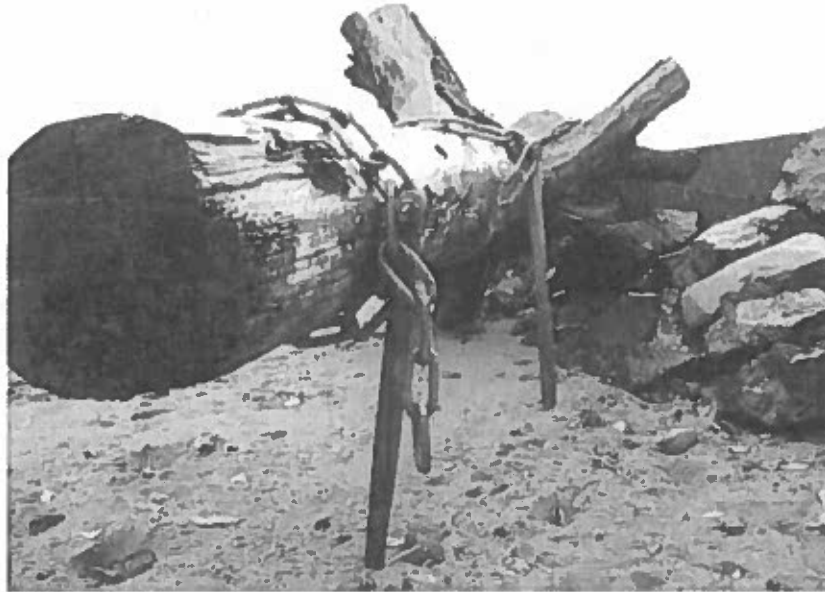
Figure 10. Anchored log shore protection structure with sand eroded from beneath Sand filled geotextile structures might be designed to remain stable in the design storm event. However, if it does not move and is not undercut, this soft solution will have about the same effect of preventing bluff erosion as a rock revetment. Because the revetment would reduce runup and rundown by its roughness and porosity and the geotextile structure would not, the soft solution could well have greater impact to the fronting beach than would the rock revetment. Geotextile is susceptible to damage by debris and vandalism.
