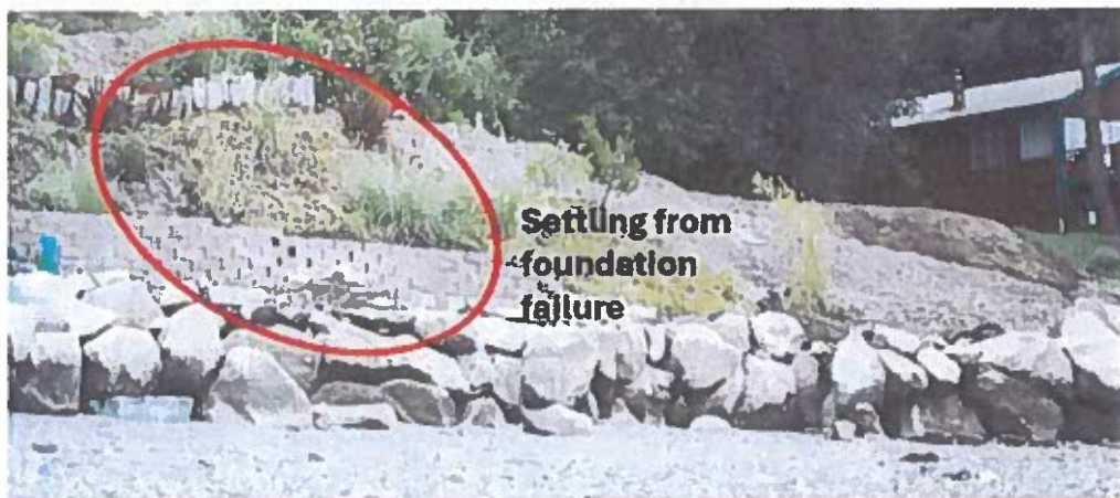
Figure 7. Settling and foundation failure from soil saturation (Fox Island, approx. 2000)
