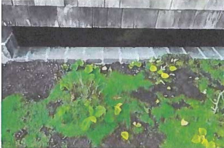
Figure 2. Ground at seaward side of Seigel residence
