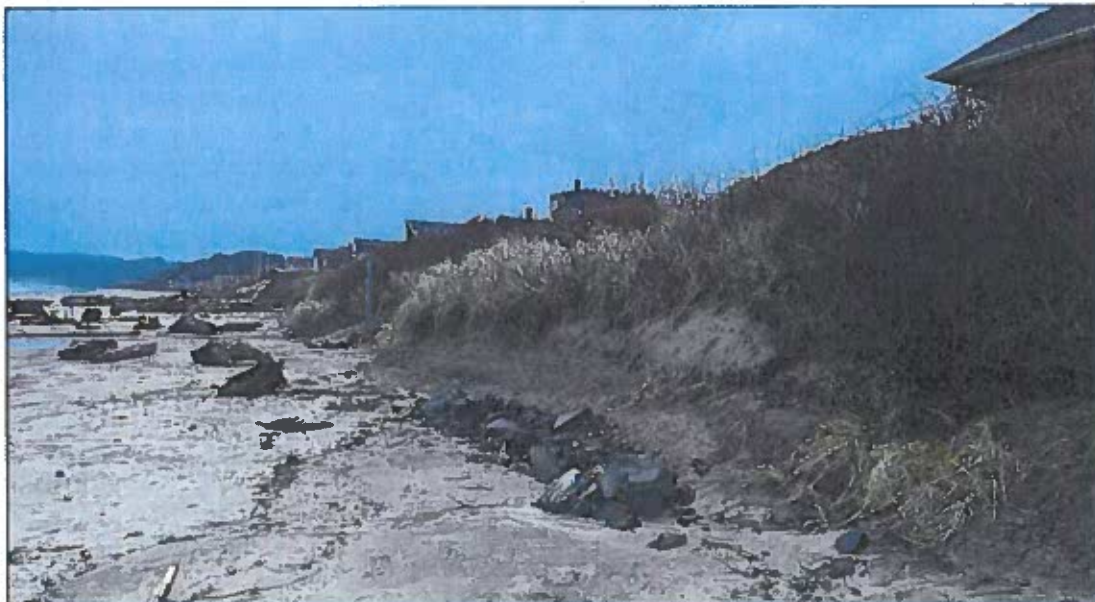
Photo 4: Site conditions at the time of a subsequent site visit on December 16, 2024, showing the continued erosion of the subject property's coastal bluff.
