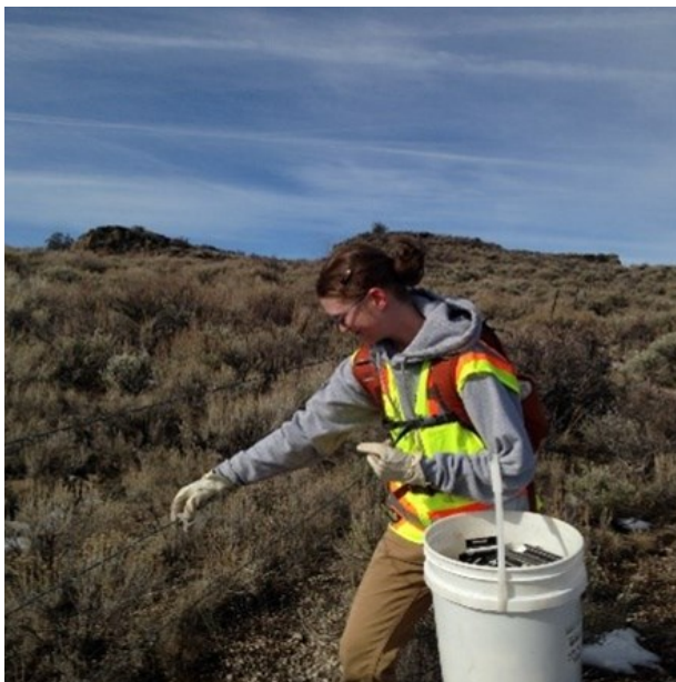
HOC AmeriCorps crews repaired range fencing located to the east of Bend. Updating old fencing improves wildlife migration, while protecting threatened and endangered species. Amber, a Land Stewardship Trainer, exhibits how to place reflectors on the wire fence.
