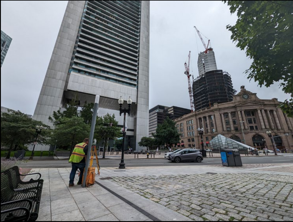
Left: A surveyor setting construction control on a new story of the building under construction in the upper right of the picture. Boston, MA for NCEES Annual Meeting.
