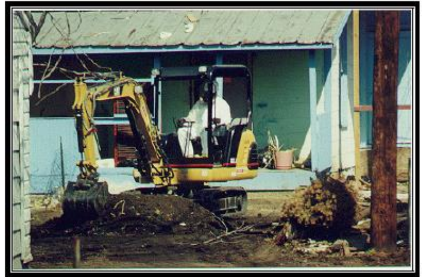
View of U.S. EPA ERRS contractor excavating mercury-contaminated soil in a residential area.
