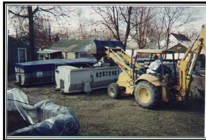
View of U.S. EPA ERRS contractor loading mercury-contaminated clothing and household items into rolloff boxes for disposal.
