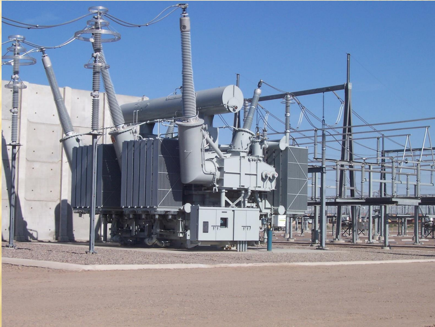
Huge-Ass Distribution Transformer, as in:
