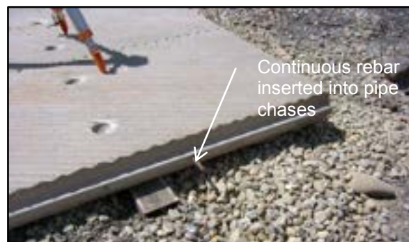
Photo 3-26 Plank with longitudinal pipe chases cast in for insertion of continuous rebar
