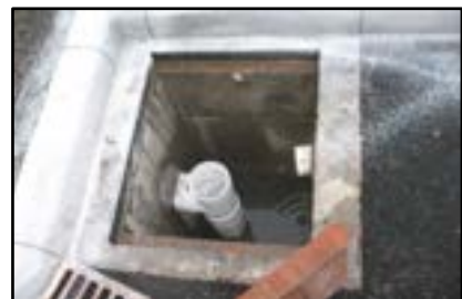
Photo 3-38 Trapped catch basin
