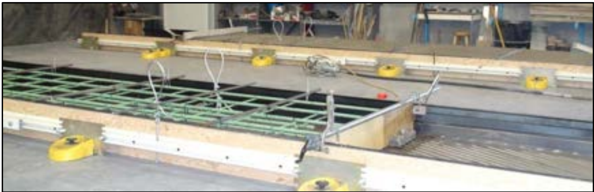
Photo 3-22 Shop fabricated precast planks. The form in the foreground is ready for placement of concrete. The form in the background has concrete in place. These planks are cast upside. The cable loops are used to lift and turn the planks and will be cut off flush with the bottom.
