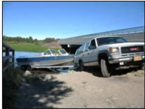
Photo 3-17 Gravel ramp in poor condition and with inadequate slope
