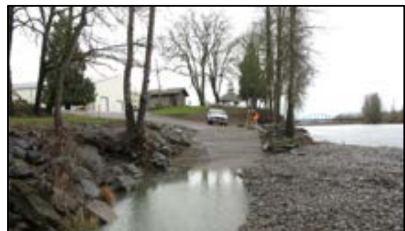
Photo 3-4 Launch ramp aligned nearly parallel to river. Development of gravel bar has made this ramp unusable at lower water levels.
