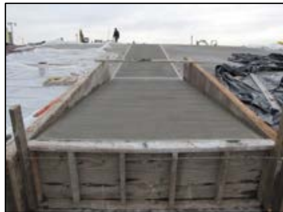
Photo 4-6 Float abutment and walkway after placement of concrete. Both have a broom finish.
