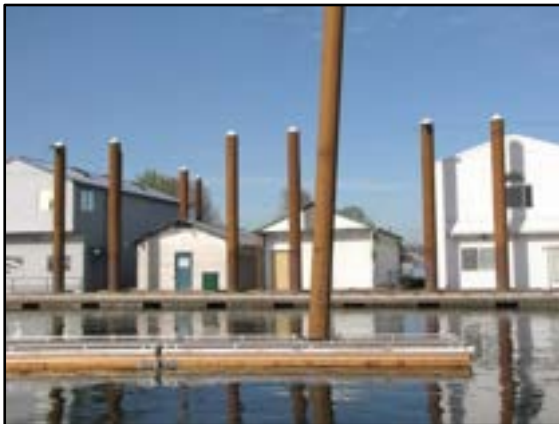
Photo 6-1 Battered boarding float pile in foreground and vertical transient float piles in background
