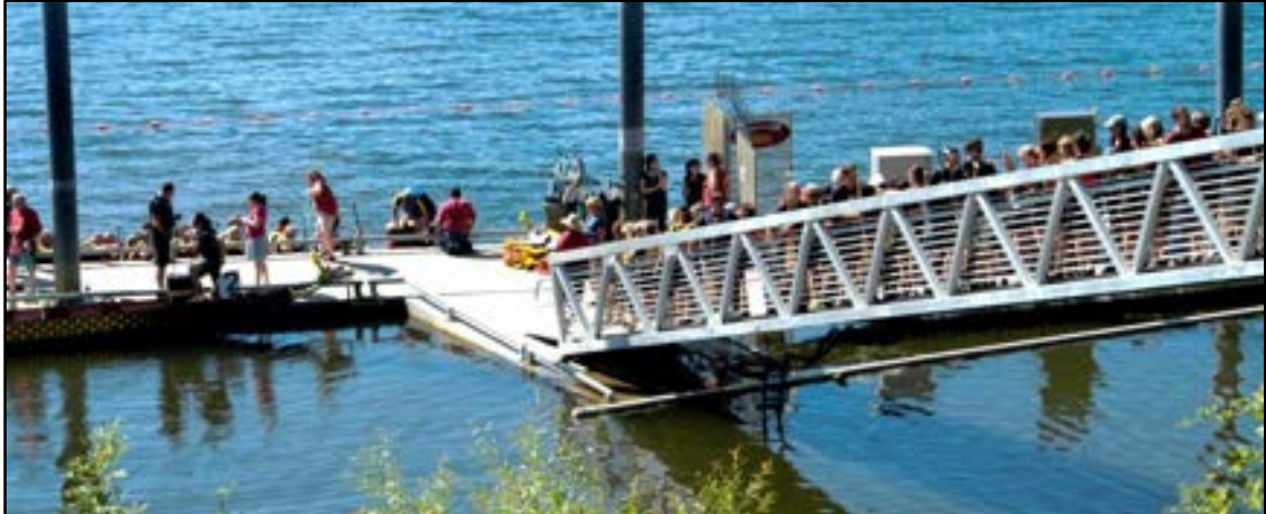
Photo 5-11 Inadequate floatation to compensate for gangway live load. Gangway support floats should be floating level under this loading condition – not submerged at shore end. Although the load is still supported this may induce stresses at the connection points and conveys a visual sense of being unsafe.
