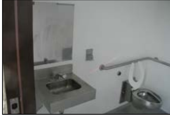
Photo 10-4 Stainless steel toilet room fixtures
