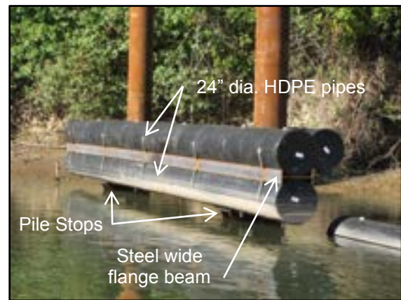
Photo 8-5 Poly-pipe debris boom details. Note pile stops to prevent grounding during low water.
