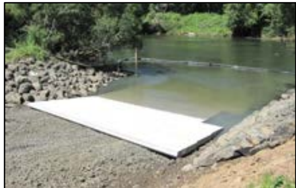
Photo 3-24 Proper number of precast planks above the water line for transition to cast-in-place ramp
