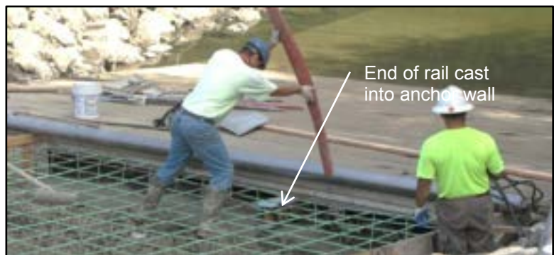
Photo 3-29 Transition from precast planks to cast-in-place concrete. This photo shows the 24" deep anchor wall being poured. A rebar pin through the web of the rail and rebar hooks into the anchor wall tie the precast planks and rail system to the cast-in-place launch ramp.
