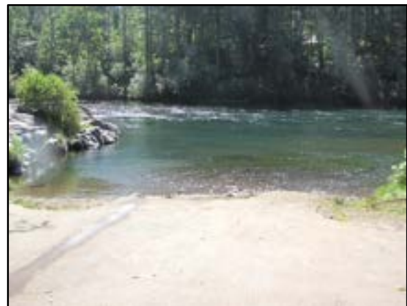
Photo 3-18 Asphalt ramp in poor condition. Note deteriorated asphalt at water's edge and missing asphalt below the water line due to inadequate edge protection and scouring from the river flow.
