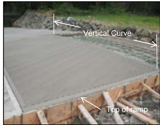
Photo 3-30 Vertical curve at top of launch ramp. Photo also shows block-out for float abutment.
