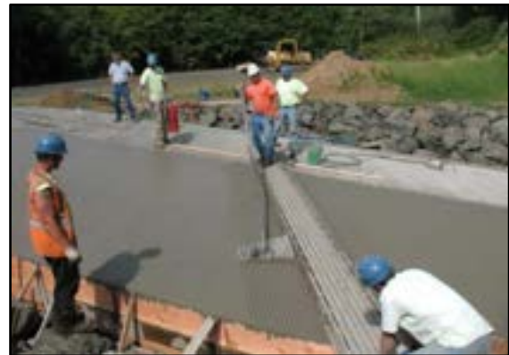
Photo 3-32 Cutting grooves into fresh concrete. The plank acts as a guide for groove alignment and tool control.
