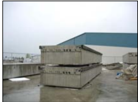
Photo 5-8 Individual float sections connected together with wood walers to make sub-assemblies. The holes in the end of the float are utility chases.
