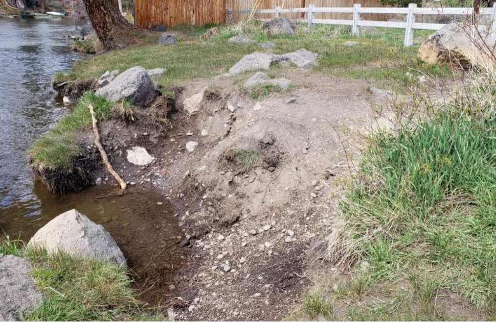
Erosion at the northern access point, which is planned to be closed as part of the project identified in the River Plan.
