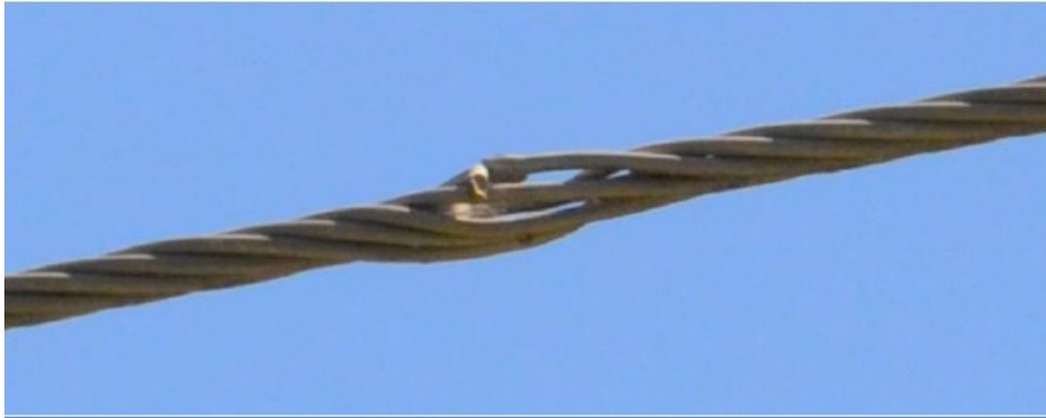
Figure 21: Damaged Conductor Identified by EFD System in 2022 and corrected by PGE
