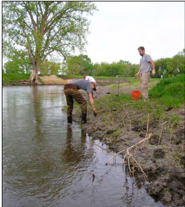
Installation of willow cuttings for revegetation of the riparian area along Elm Creek, Minnesota. Photo Credit: Britta Suppes, Joe Magner, Chris Lenhart
