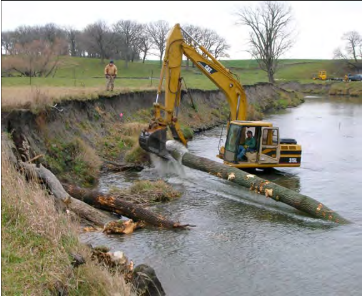
Installation of log vanes and a bankfull bench on Elm Creek, Minnesota in the southern glaciated cornbelt region. Photo Credit: Britta Suppes, Joe Magner, Chris Lenhart
