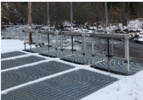
Headworks diversion gates to be updated at Sheirbon Hill Water Conservation Project.
