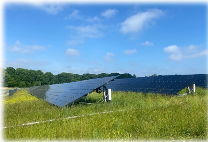
Figure 2 - A 4 MW landfill solar project in Cuyahoga County, Ohio.
