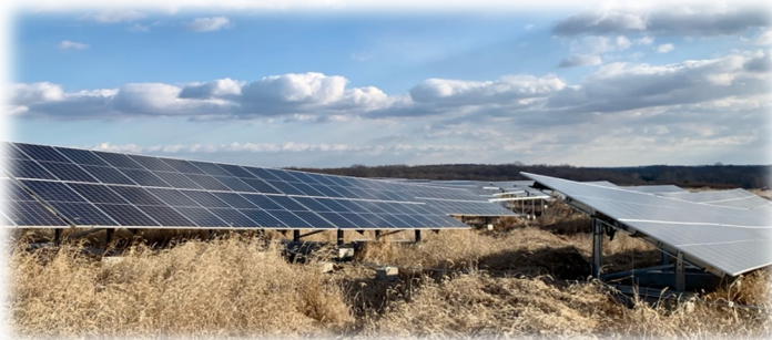
Figure 1 - A 6 MW community solar project on a closed landfill in Montgomery County, Maryland.
