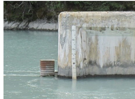
Figure 9. Staff plates in a reservoir. (Credit: National Weather Service)
