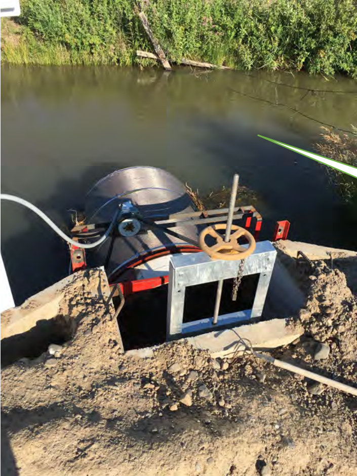
Screen and headgate
