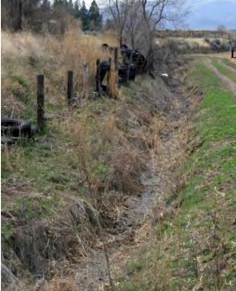
Dirt canals are susceptible water loss through leakage and evaporation.
