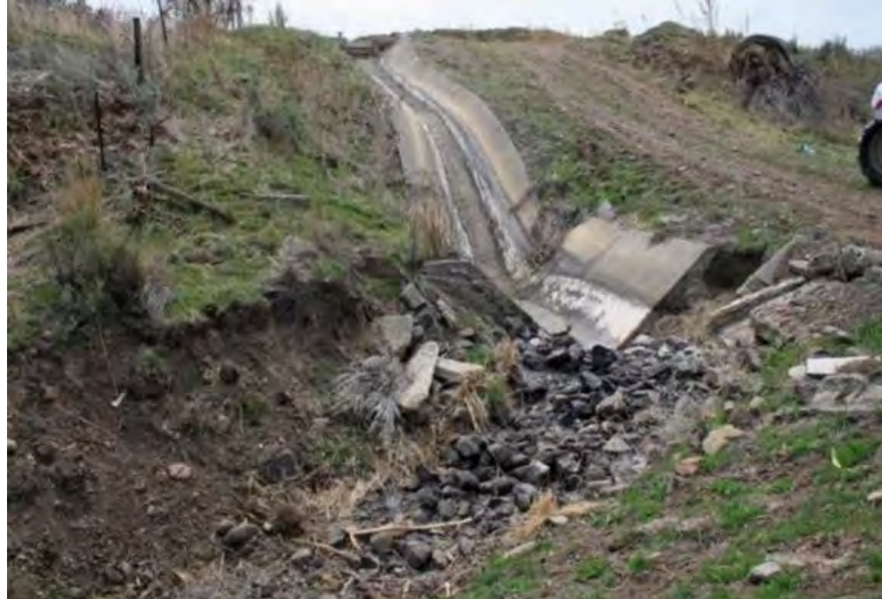
Typical spillway. Note the erosion of the ditch.
