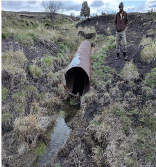
Figure 11. An undersized culvert abandoned instream. Site location where one of six hardened water crossing will be constructed livestock to cross without impacting creek.
