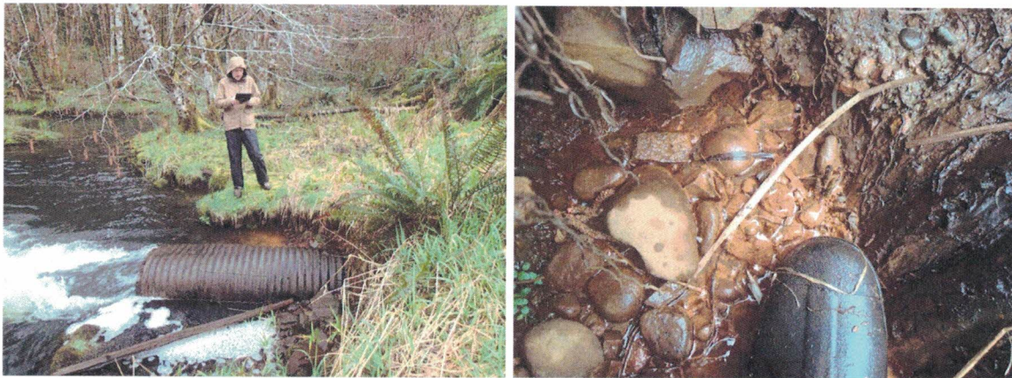
30 inch diameter corrugated metal pipe conduit with seepage
