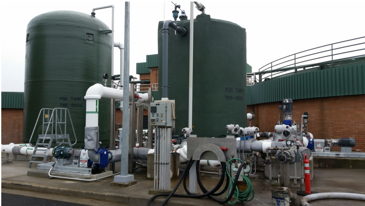
FOG RECEIVING STATION
