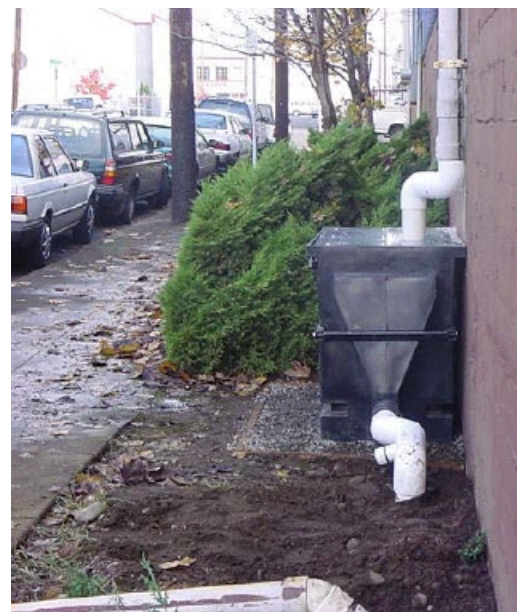
Roof Downspout type filter
