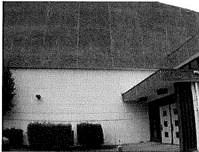
E Falling Hazard
