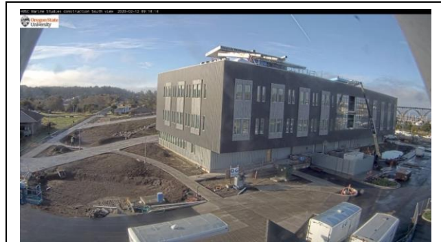
Figure 2. The construction of the new tsunami resistant building nearing completion. Accessed on February 12, 2020 from http://hubsum.oregonstate.edu/sum/sumsouth/live/live.jsp
