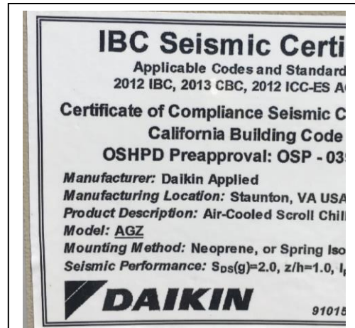
Figure 2. This hospital chiller equipment has been tested to perform well after earthquake shaking and has a “seismically certified” label.
